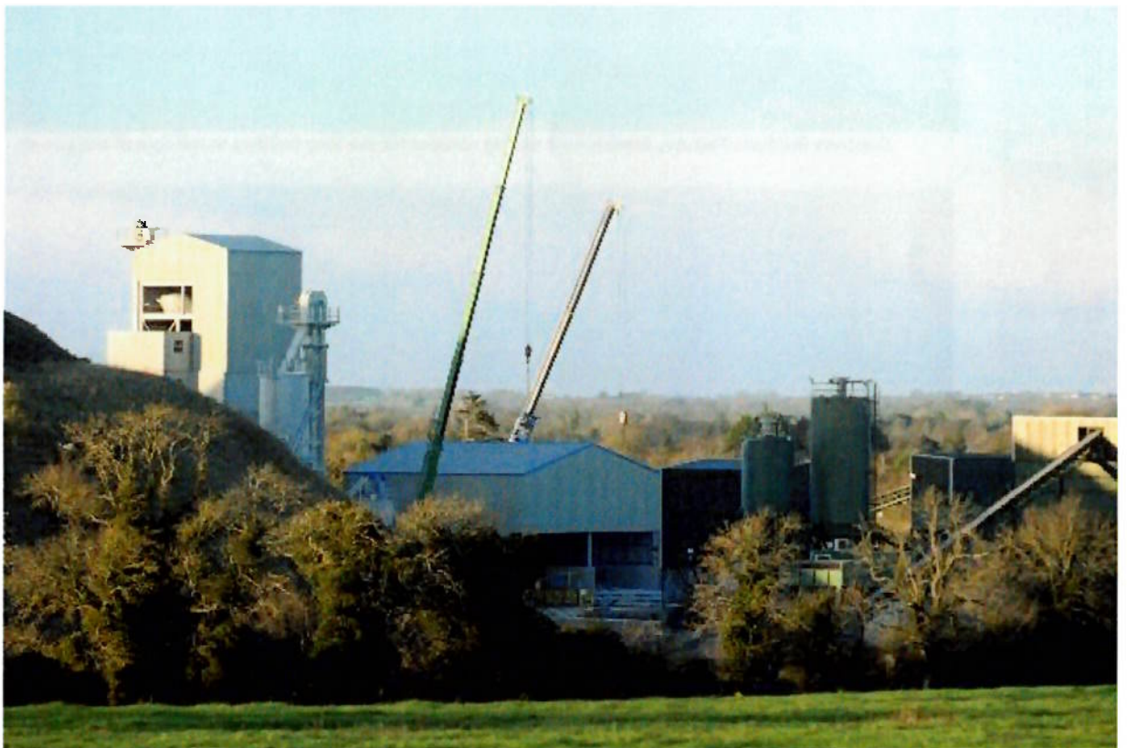
Construction of plant in 2016 without planning consent
